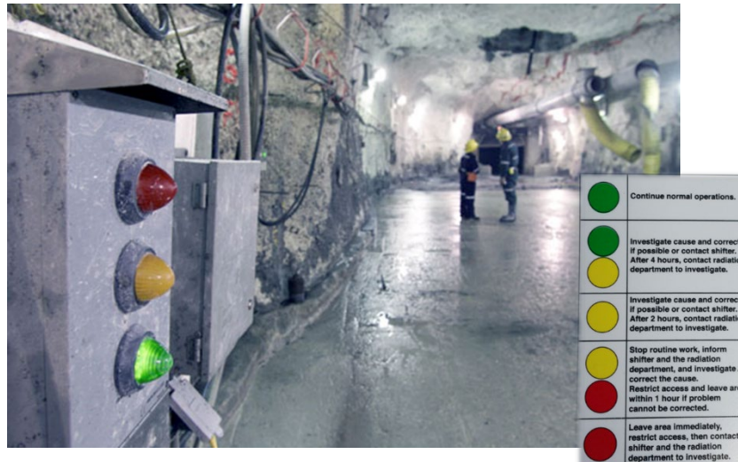
Fig. 2. An image of a continuous radon progeny monitor and quick reference guide to key actions in the Code of Practice.
